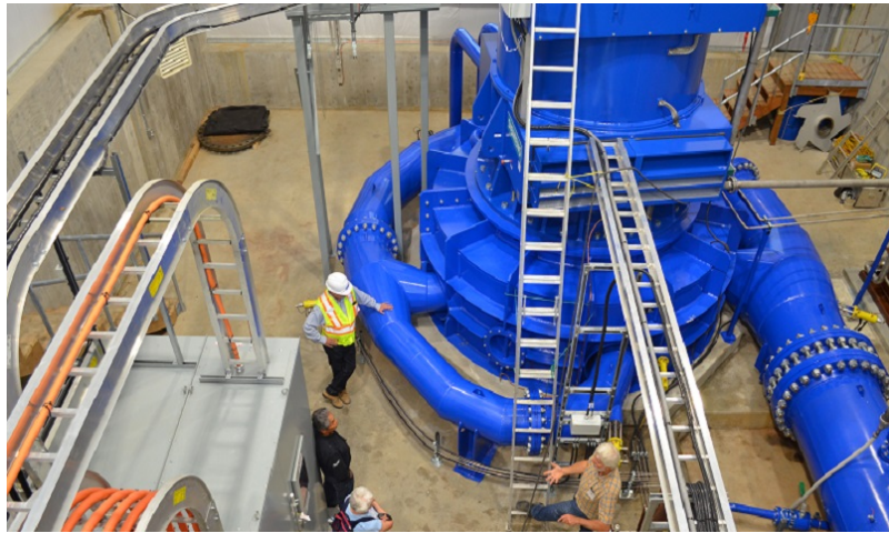
Powerhouse at Winchie Creek Hydro
