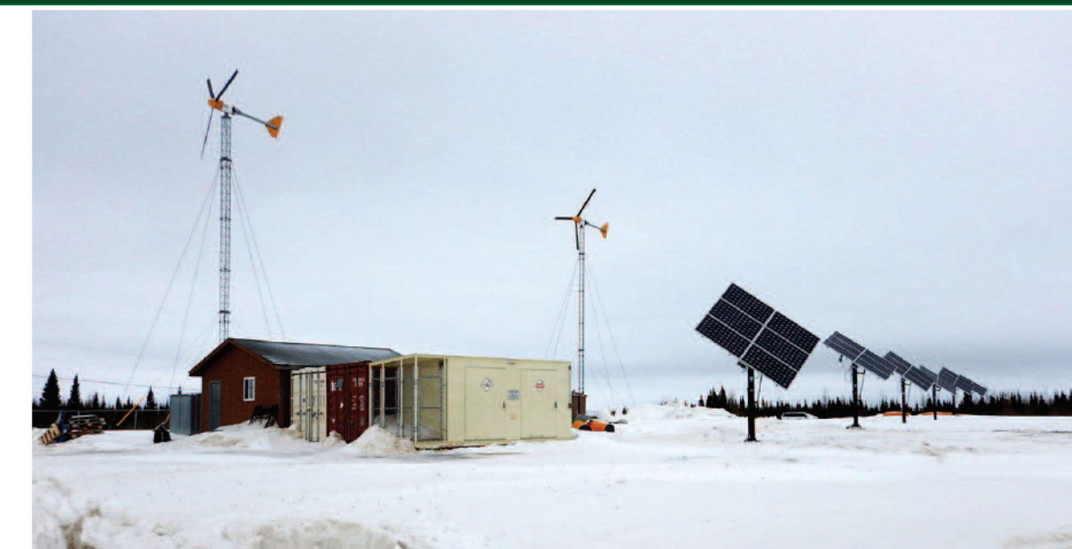
A small wind-solar facility installed at the airport of the remote community of Peawanuck in Ontario [4]
